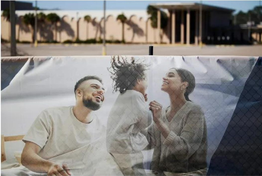
Advertising hangs on a fence line promoting the Village at Town Center Wednesday, Feb. 1, 2023 at the Morocco Shrine Center in Jacksonville, Fla. The Klotz Group of Companies and KABR Group begin demolition of the former active Morocco Shrine Center, a city landmark for 36 years and one of Jacksonville's iconic fixtures. The building is being torn down to make way for the new Village at Town Center. The project will span 37 acres and be home to 1,025 units that include high-end luxury residential and student housing, plus 115,00 square feet of retail, restaurant, and office space. Corey Perrine/Florida Times-Union
